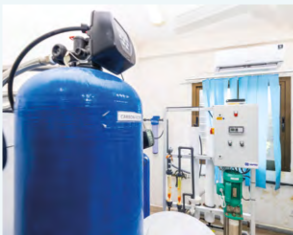
Reverse osmosis system at an AHN Clinic in Tanzania
